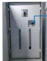
CB Rating: 600AT (Supplying Firepump) Location: Bldg.5, Ground Floor EE Room
