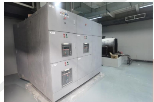
SYNCHRO PANELS & SWITCHGEARS
