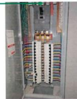
CB Rating: 400AT (Supplying 6F) Location: Bldg.5, 6th Floor EE Room
