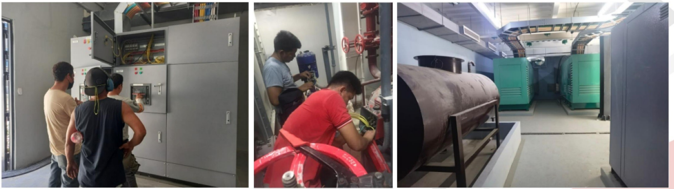
SUPPLY AND INSTALLATION OF GENERATOR SETS, SYNCHRONIZING PANEL, ATS AND OTHER ELECTRICAL EQUIPMENTS PHASE 1R IC MIXED USE PROJECT, KAWIT CAVITE
